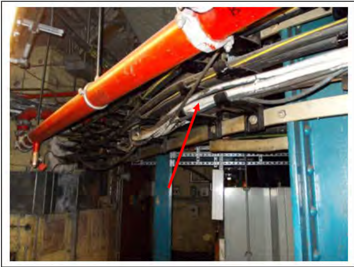
FIGURE 5: STRONGLY PRESUMED ASBESTOS IN CLOTH CABLE WRAP UMC ACCESS, 2/151 - DESCRIPTION & RESULT OF ASSESSMENT (SAMPLE REF. SP1(5))
