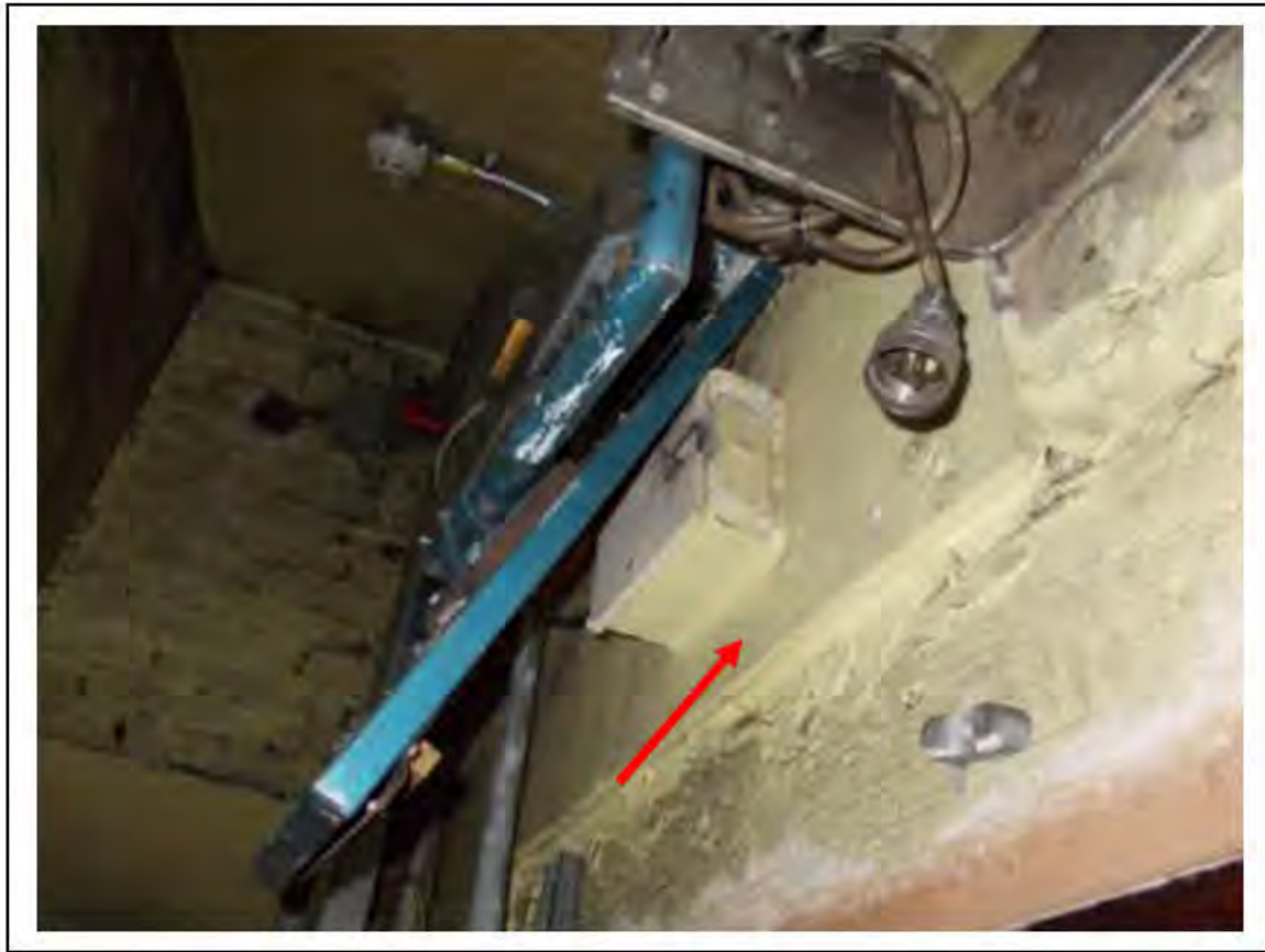
FIGURE 15: STRONGLY PRESUMED ASBESTOS IN INSULATION BOARD IN UMC ACCESS, 3/152 - DESCRIPTION & RESULT OF ASSESSMENT (SAMPLE REF. SP2(1))
