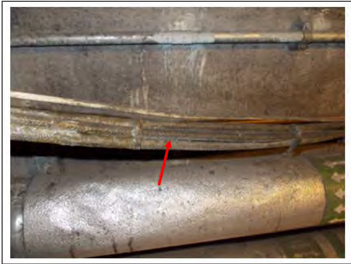
FIGURE 12: STRONGLY PRESUMED ASBESTOS IN CLOTH CABLE WRAP UMC ACCESS, 3/151 - DESCRIPTION & RESULT OF ASSESSMENT (SAMPLE REF. SP1(9))
