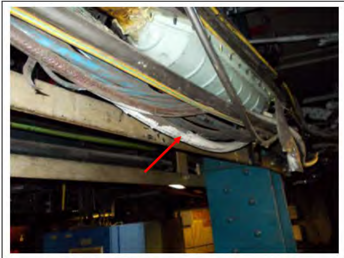
FIGURE 6: STRONGLY PRESUMED ASBESTOS IN CLOTH CABLE WRAP UMC ACCESS, 2/151 - DESCRIPTION & RESULT OF ASSESSMENT (SAMPLE REF. SP1(6))
