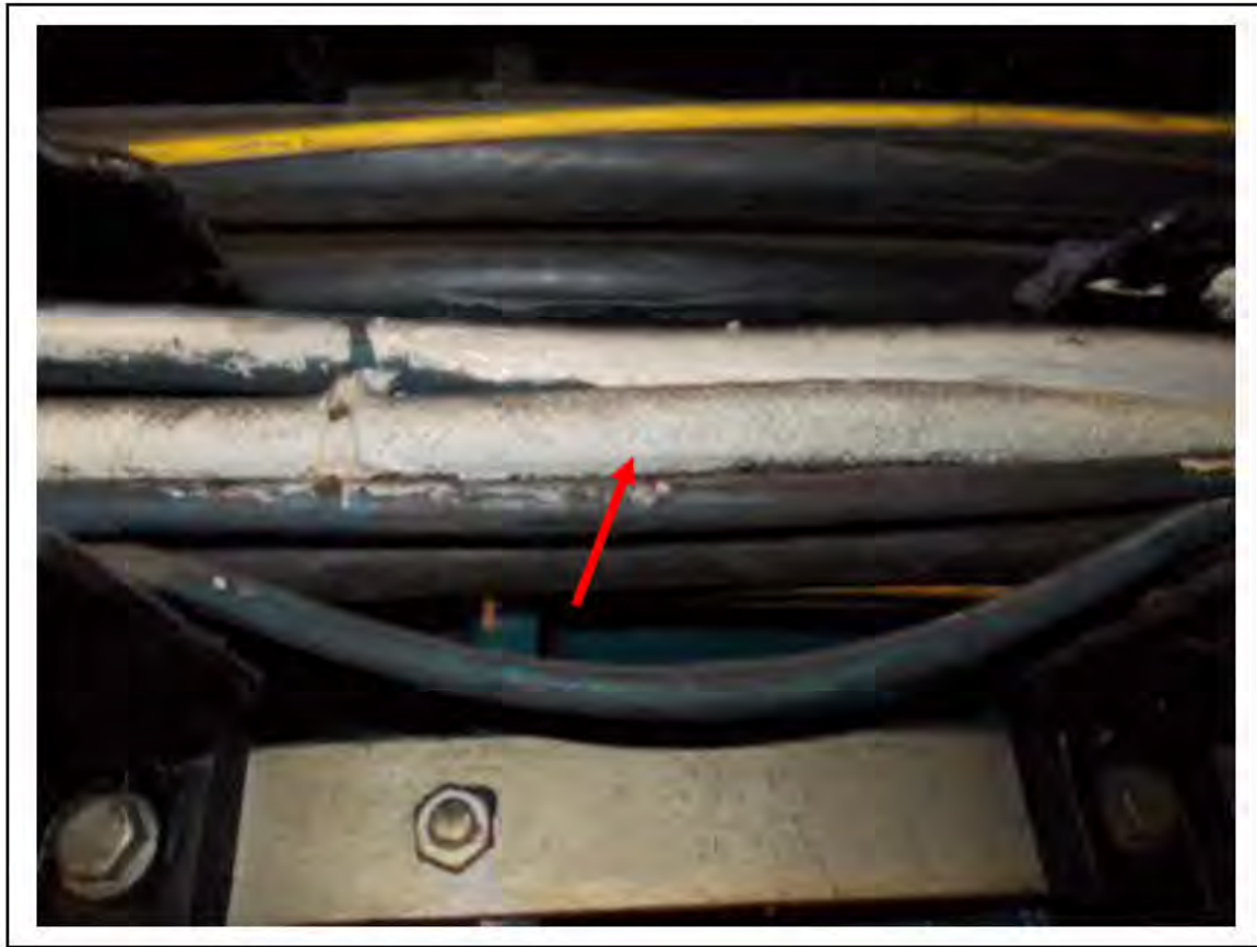
FIGURE 22: CONFIRMED ASBESTOS IN ASBESTOS CLOTH IN RELAY ROOM, 5/711 - DESCRIPTION & RESULT OF ASSESSMENT (SAMPLE REF. ECS 81549)
