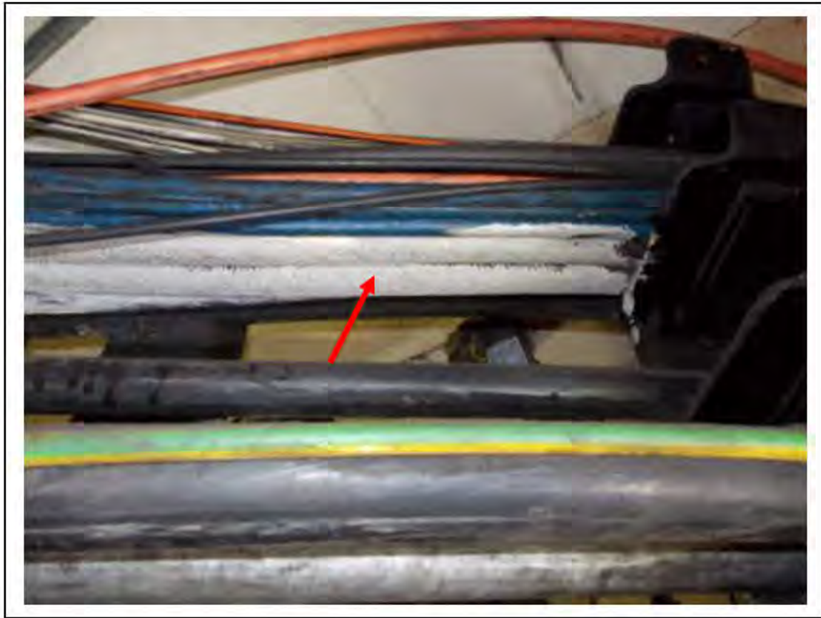
FIGURE 25: STRONGLY PRESUMED ASBESTOS IN CLOTH CABLE WRAP LMC ACCESS, 6/161 - DESCRIPTION & RESULT OF ASSESSMENT (SAMPLE REF. SP1(15))
