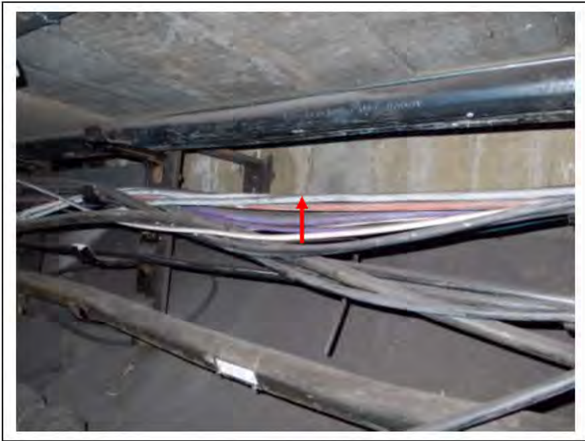
FIGURE 33: STRONGLY PRESUMED ASBESTOS IN CLOTH CABLE WRAP CABLE DUCT, 6/786 - DESCRIPTION & RESULT OF ASSESSMENT (SAMPLE REF. SP1(20))
