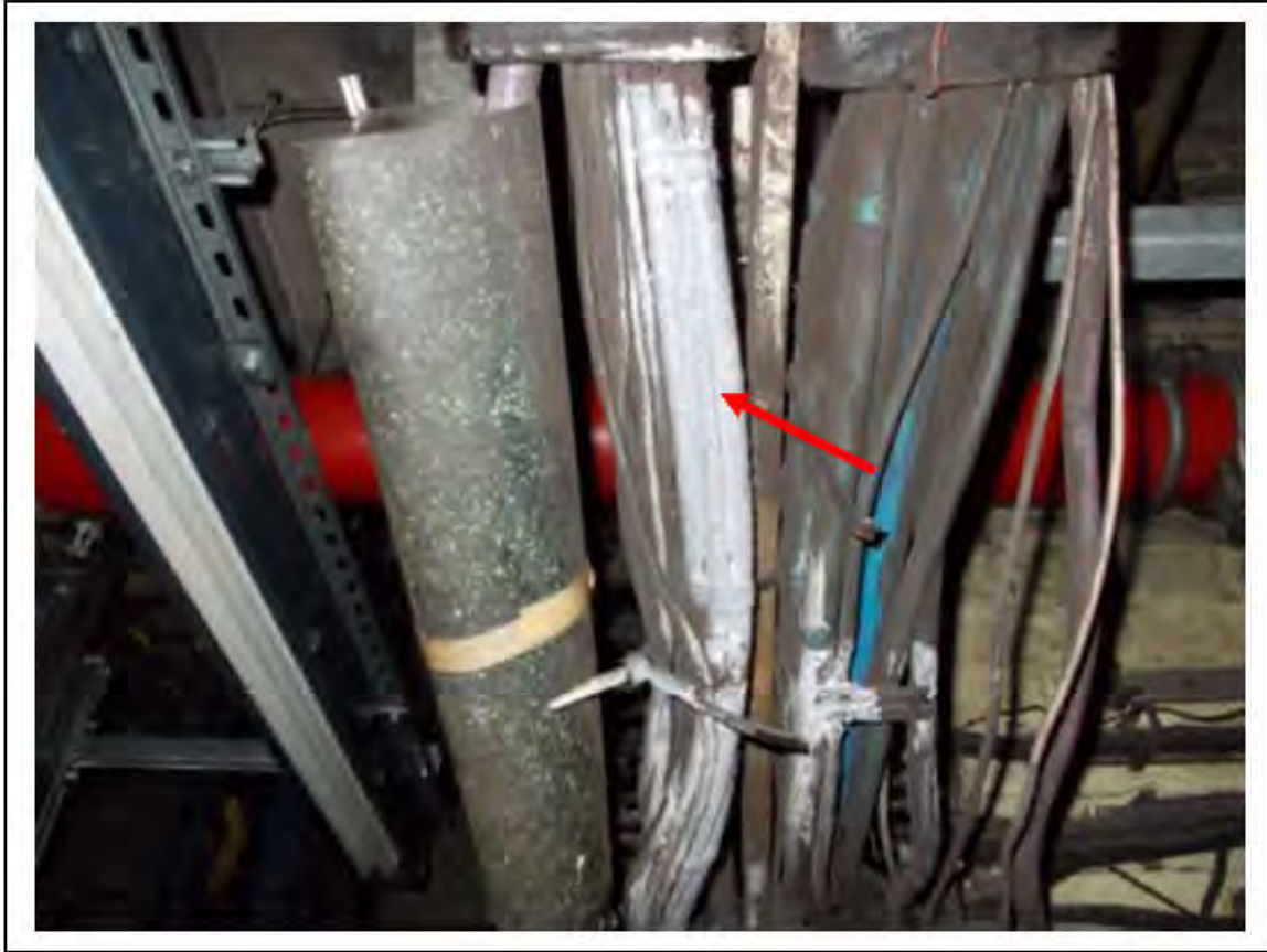
FIGURE 4: STRONGLY PRESUMED ASBESTOS IN CLOTH CABLE WRAP UMC ACCESS, 2/151 - DESCRIPTION & RESULT OF ASSESSMENT (SAMPLE REF. SP1(4))
