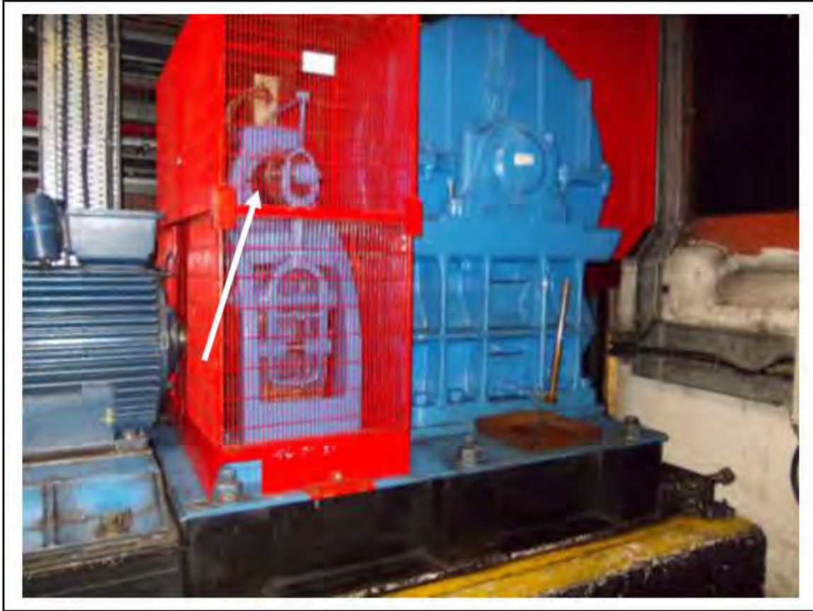
FIGURE 8: STRONGLY PRESUMED ASBESTOS IN BRAKE PADS IN UMC ACCESS, 2/151 - DESCRIPTION & RESULT OF ASSESSMENT (SAMPLE REF. SP1(1))
