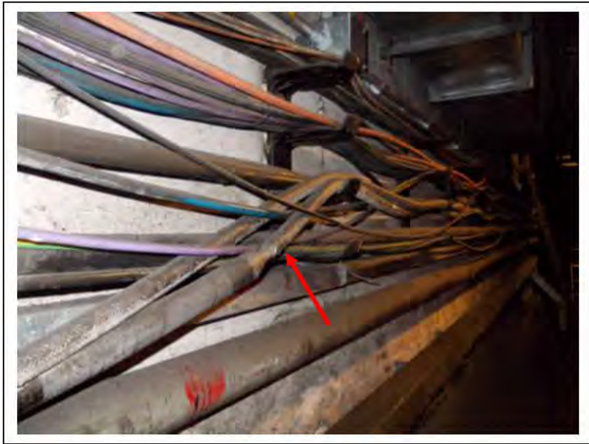
FIGURE 13: STRONGLY PRESUMED ASBESTOS IN CLOTH CABLE WRAP UMC ACCESS, 3/151 - DESCRIPTION & RESULT OF ASSESSMENT (SAMPLE REF. SP1(10))
