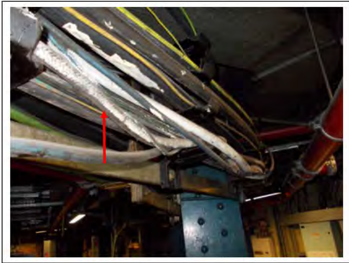
FIGURE 30: STRONGLY PRESUMED ASBESTOS IN CLOTH CABLE WRAP RELAY ROOM, 6/713 - DESCRIPTION & RESULT OF ASSESSMENT (SAMPLE REF. SP1(17))
