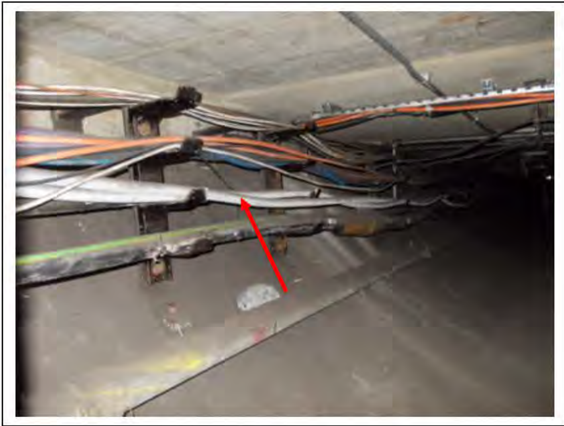
FIGURE 27: STRONGLY PRESUMED ASBESTOS IN CLOTH CABLE WRAP CABLE DUCT, 6/787 - DESCRIPTION & RESULT OF ASSESSMENT (SAMPLE REF. SP1(21))
