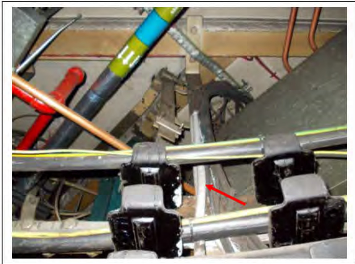
FIGURE 2: STRONGLY PRESUMED ASBESTOS IN CLOTH CABLE WRAP UMC ACCESS, 2/151 - DESCRIPTION & RESULT OF ASSESSMENT (SAMPLE REF. SP1(2))
