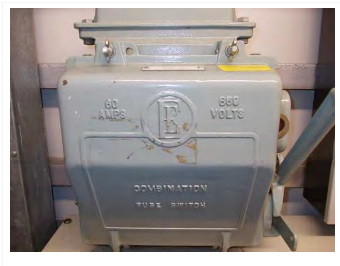
FIGURE 18: POSSIBLE ACMS WITHIN SWITCHGEAR IN PUMP ROOM, 3/776 - DESCRIPTION & RESULT OF ASSESSMENT (SAMPLE REF. P1(4))
