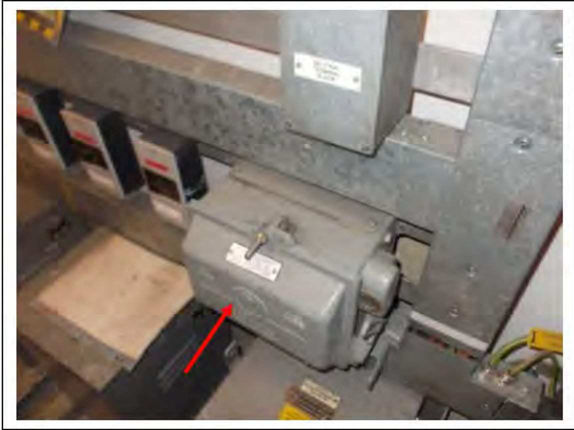
FIGURE 1: POSSIBLE ACMS WITHIN SWITCH GEAR IN SWITCH ROOM, 1/662 - DESCRIPTION & RESULT OF ASSESSMENT (SAMPLE REF. P1(1))
