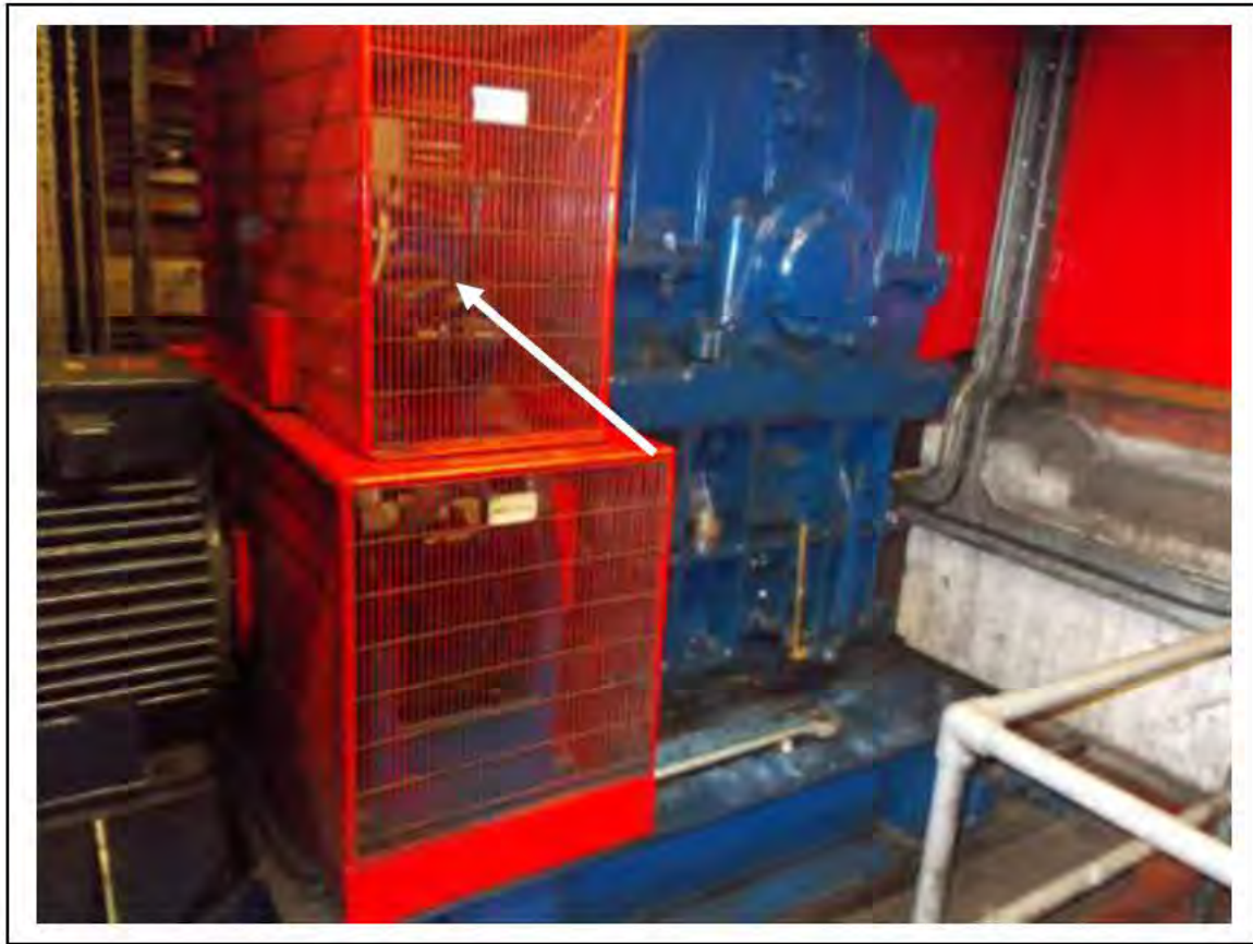
FIGURE 14: STRONGLY PRESUMED ASBESTOS IN BRAKE PADS IN UMC ACCESS, 3/151 - DESCRIPTION & RESULT OF ASSESSMENT (SAMPLE REF. SP1(11))
