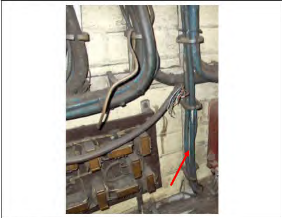
FIGURE 32: STRONGLY PRESUMED ASBESTOS IN CLOTH CABLE WRAP CER, 6/731 - DESCRIPTION & RESULT OF ASSESSMENT (SAMPLE REF. SP1(19))
