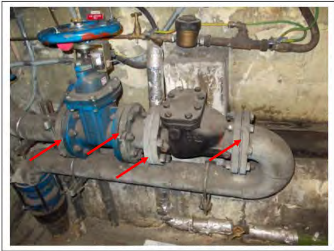
FIGURE 7: CONFIRMED ASBESTOS IN ASBESTOS GASKET IN UMC ACCESS, 2/151 - DESCRIPTION & RESULT OF ASSESSMENT (SAMPLE REF. ECS 81597)
