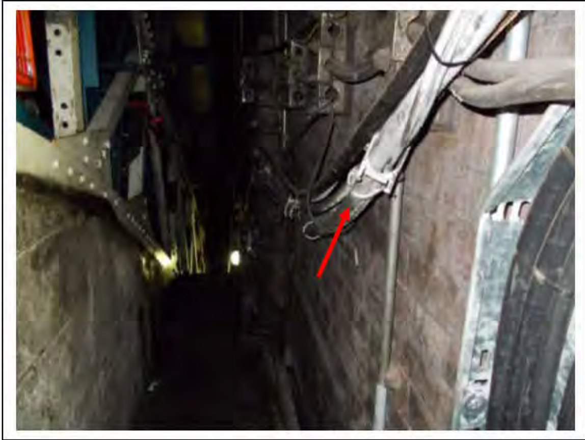
FIGURE 9: STRONGLY PRESUMED ASBESTOS IN WOVEN CABLE SHEATH IN ESC SHAFT, 2/171 - DESCRIPTION & RESULT OF ASSESSMENT (SAMPLE REF. SP1(7))
