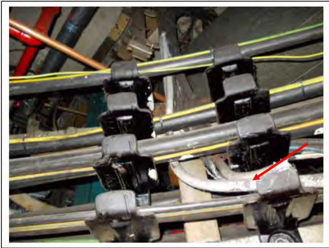
FIGURE 3: STRONGLY PRESUMED ASBESTOS IN CLOTH CABLE WRAP UMC ACCESS, 2/151 - DESCRIPTION & RESULT OF ASSESSMENT (SAMPLE REF. SP1(3))
