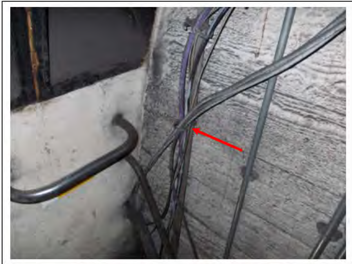
FIGURE 21: STRONGLY PRESUMED ASBESTOS IN WOVEN CABLE IN ACCESS TO LMC, 4/161 - DESCRIPTION & RESULT OF ASSESSMENT (SAMPLE REF. SP1(13))
