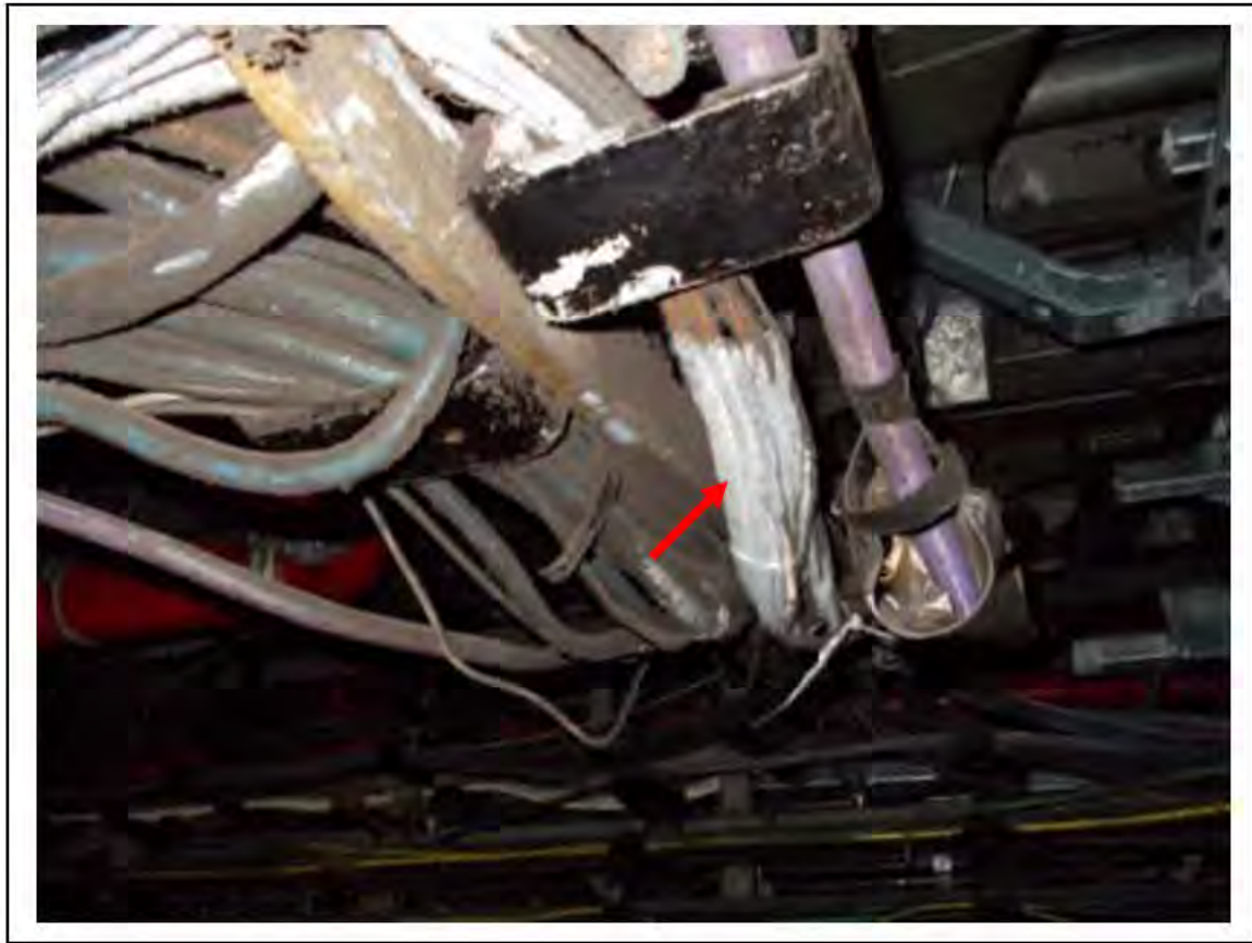
FIGURE 31: STRONGLY PRESUMED ASBESTOS IN CLOTH CABLE WRAP RELAY ROOM, 6/714 - DESCRIPTION & RESULT OF ASSESSMENT (SAMPLE REF. SP1(18))
