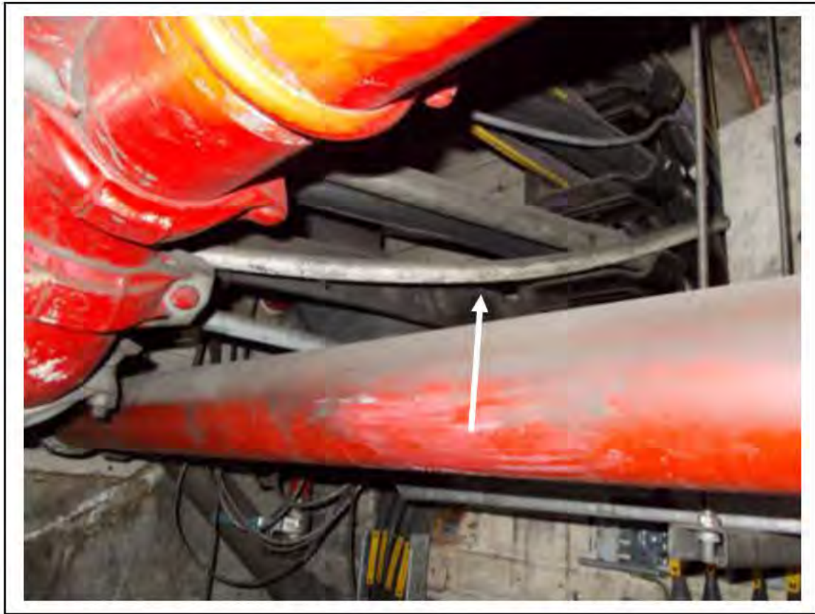
FIGURE 11: STRONGLY PRESUMED ASBESTOS IN CLOTH CABLE WRAP UMC ACCESS, 3/151 - DESCRIPTION & RESULT OF ASSESSMENT (SAMPLE REF. SP1(8))
