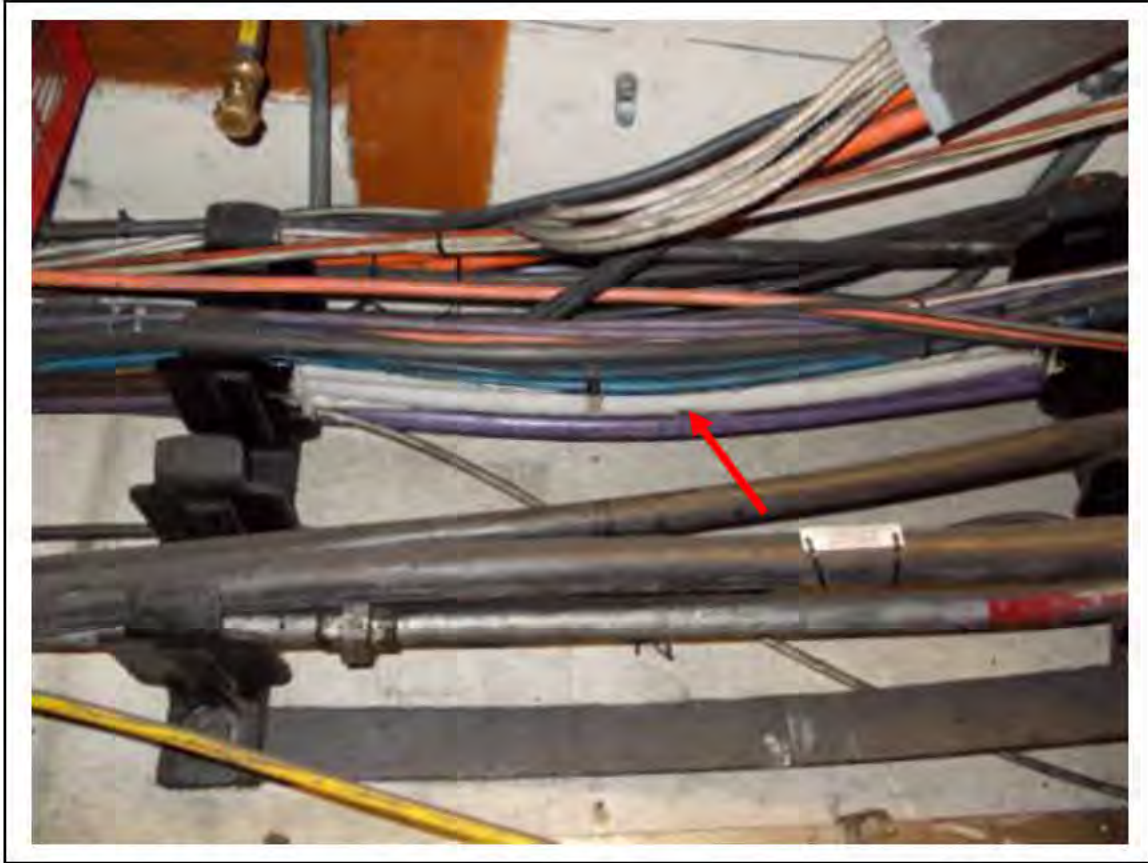
FIGURE 28: STRONGLY PRESUMED ASBESTOS IN CLOTH CABLE WRAP RELAY ROOM, 6/711 - DESCRIPTION & RESULT OF ASSESSMENT (SAMPLE REF. SP1(16))
