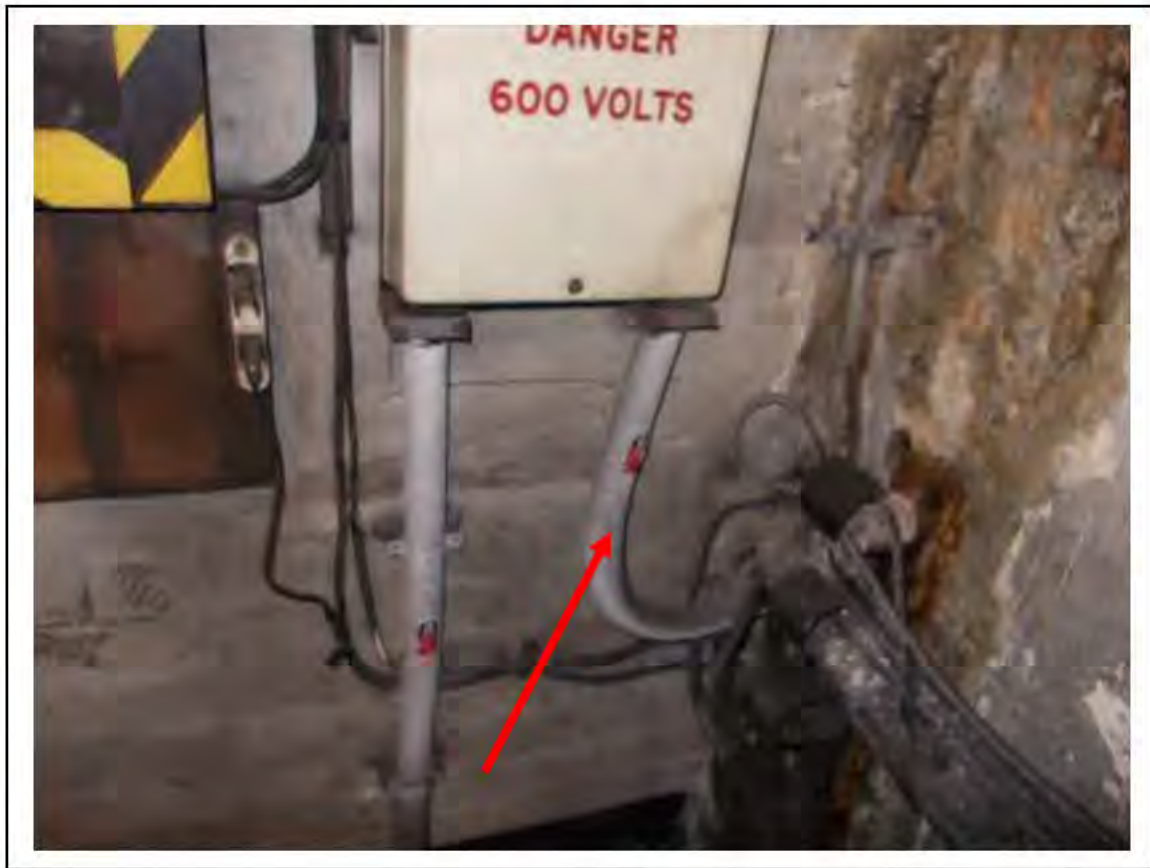
FIGURE 34: CONFIRMED ASBESTOS IN CLOTH CABLE WRAP RELAY ROOM 5/712 - DESCRIPTION & RESULT OF ASSESSMENT (SAMPLE REF. ECS 81541)
