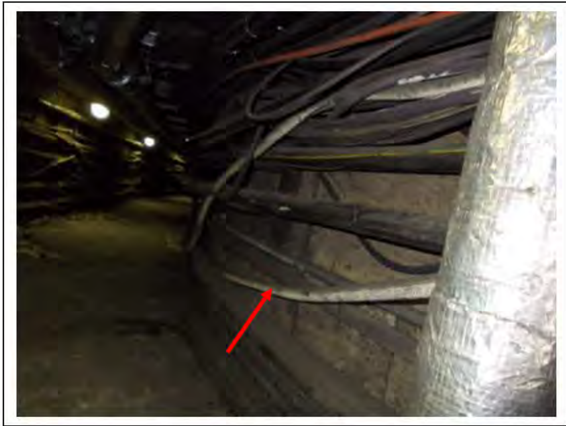
FIGURE 20: STRONGLY PRESUMED ASBESTOS IN CLOTH WOVEN CABLE SHEATH IN CABLE DUCT, 3/786 - DESCRIPTION & RESULT OF ASSESSMENT (SAMPLE REF. SP1(23))
